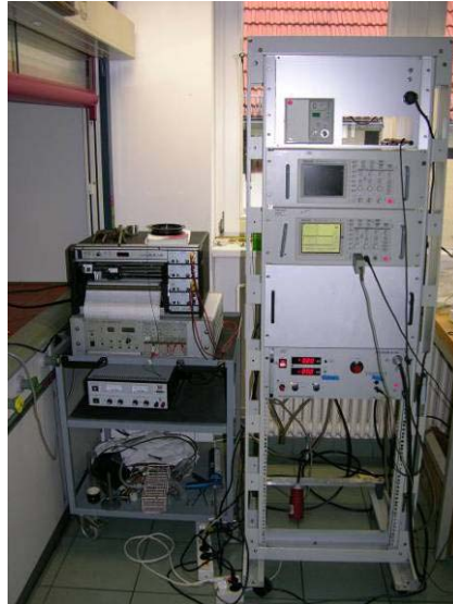
Figure 3.2: Pulse modulator with 16 kV peak voltage and 100 J/s average power (right rack) and fibre optic temperature measurement unit (left).
